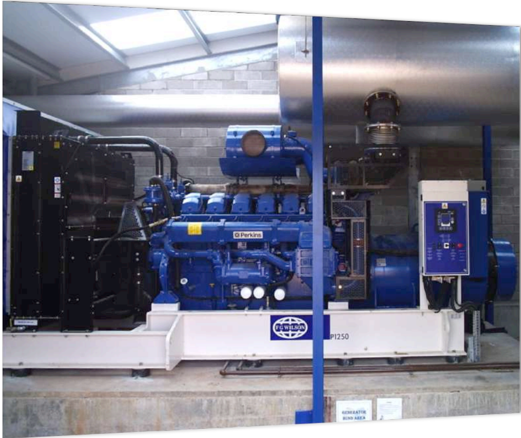
1200 kW Diesel Generator
